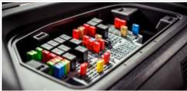
In-cab electrical panel
